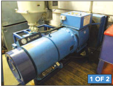
COMPAIR 50 HP Air compressors
