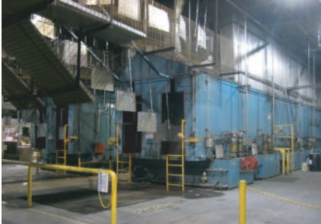
Dual Wash Line & Ovens
