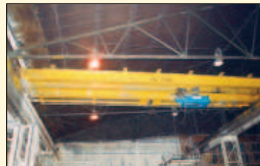
15-Ton Overhead Bridge Crane
