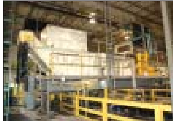
Barnes 1,800 GPM Water Soluble Coolant/2,200 LB Aluminum Chips/Hour Central Coolant System
