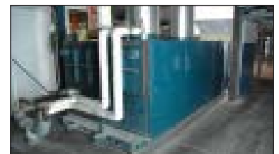
Underwriters Laboratory Natural Gas Fired Boiler System
