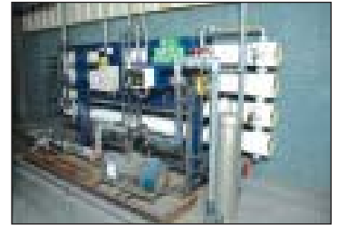
U.S. Filter System Company Water System
