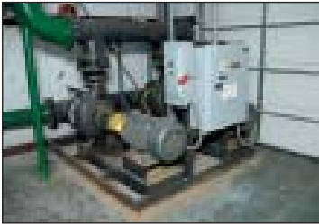
Berrington Skid Mounted Cooling Tower Water Pump System
