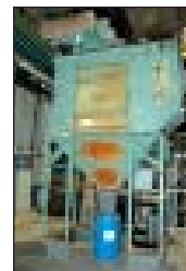
Deep Dbl. Shot Blast Room w/BCP Dust Collection Sys.
