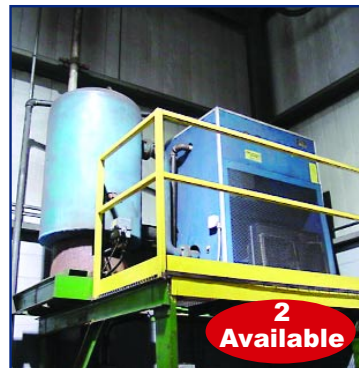
ZURN 375 CFM COMPRESSED AIR DRYER, MDL. 75R-75A
