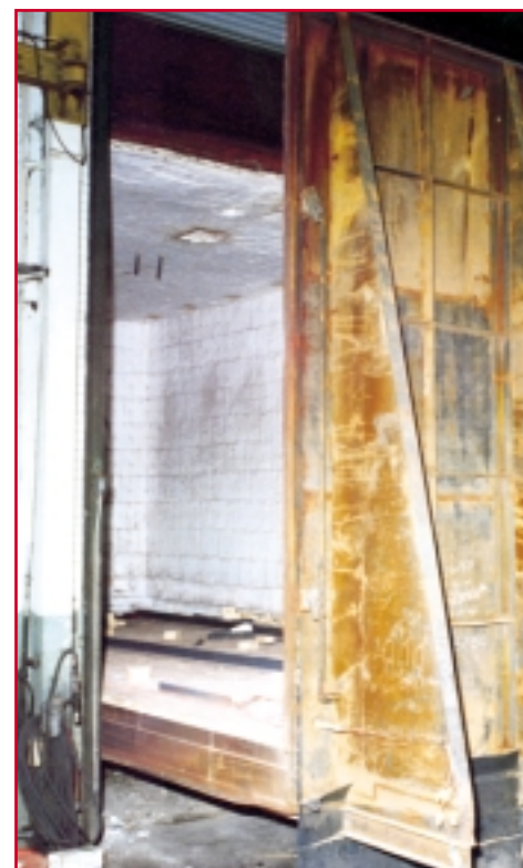
Car Bottom Furnace
