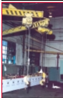
View of Jib Cranes
