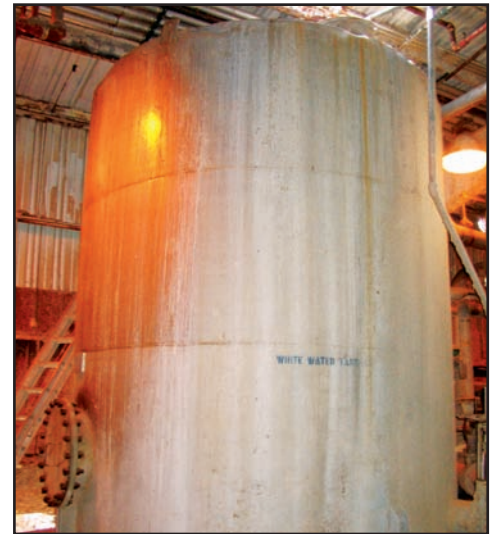
Stainless Steel Tanks
