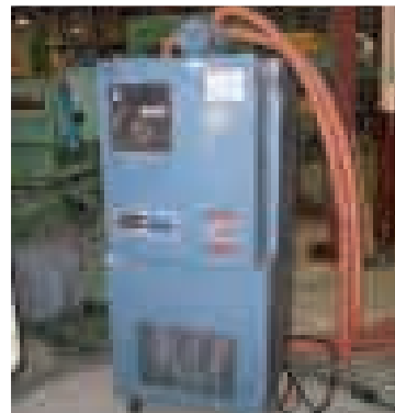
AEC Whitlock Dryer Control
