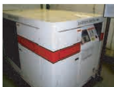
Gardner Denver 50 HP Compressor
