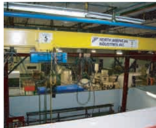
5 Ton North American Industries Bridge Crane
