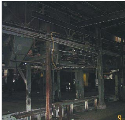
G STATION OVERHEAD SAND SYSTEM
