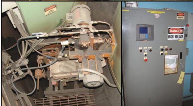
Simpson Mdl. 22G Multimull Sand Muller (Foundry D) Dietert Compactability Controller w/Panel
