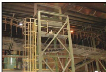
Cork Casting Monorail Chain Conveyor System
